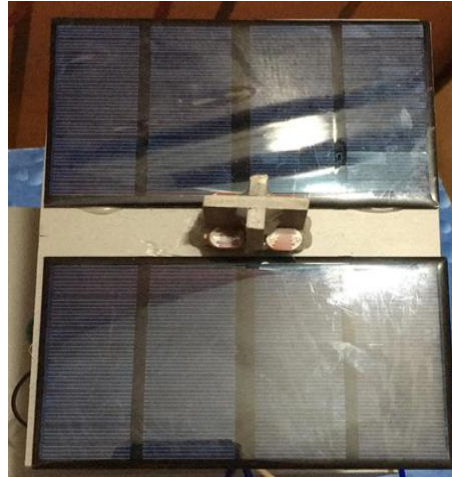
Fig. 10. PV panels and LDRs
